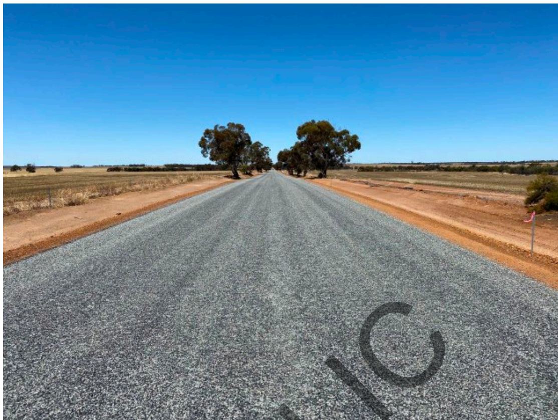
Final sealing of Yerecoin SE Rd for 2km after Reconstruction in early November 2020
