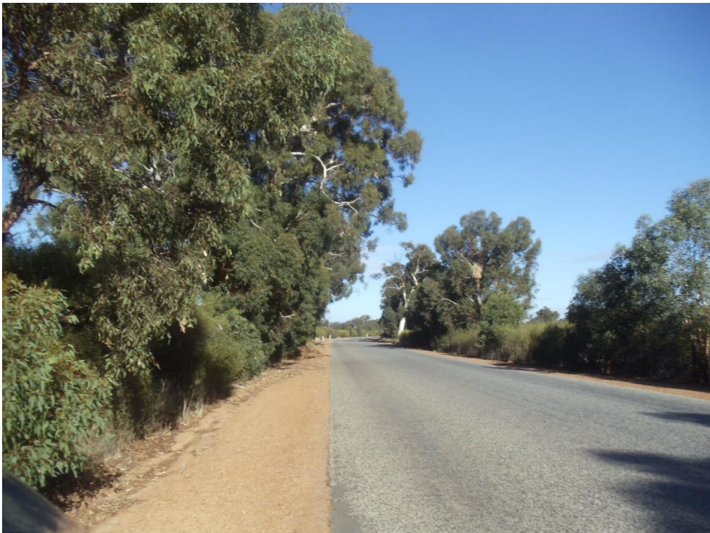
Looking west at start of right hand curve – note narrow gravel shoulder
