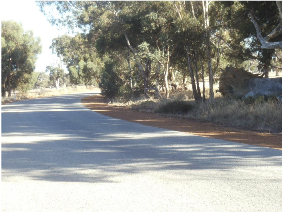
Looking west through right hand curve – note lack of sight distance - unsafe
