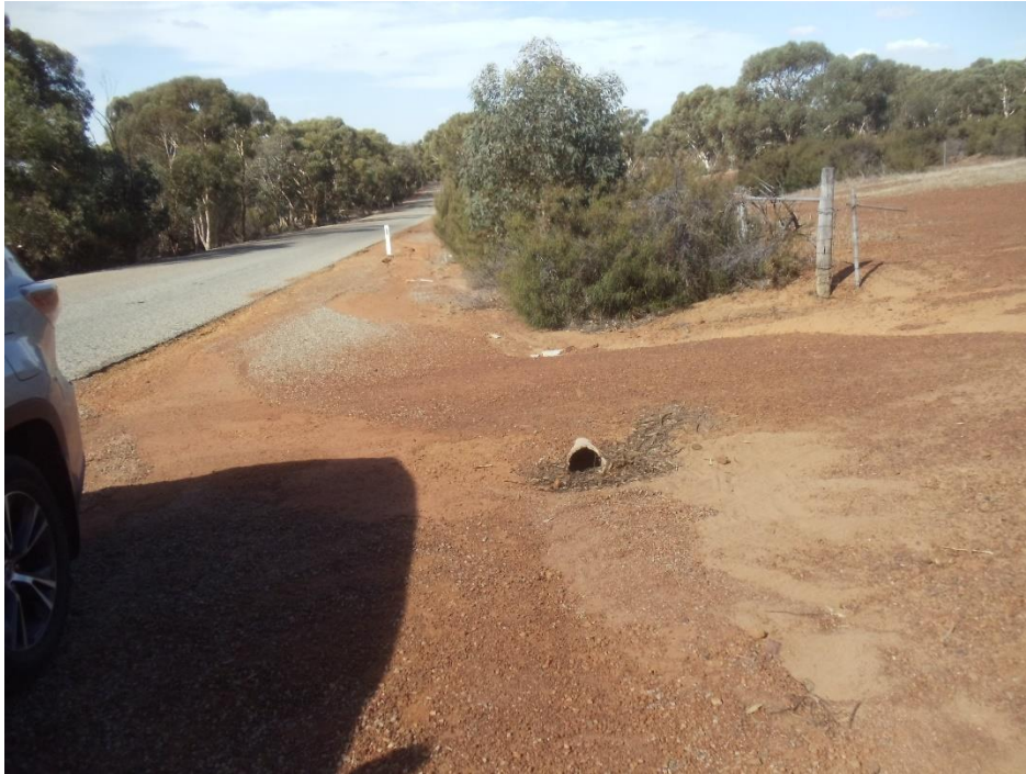
Poor drainage on southern side of road
