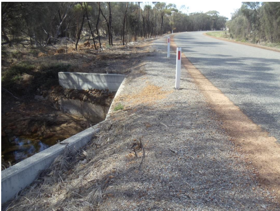
Shoulder on north side of road - narrow
