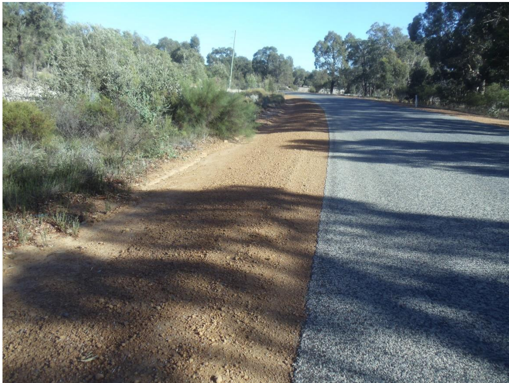
Note trucks running off road on inside of curve – narrow shoulder encroachment of vegetation on right hand side
