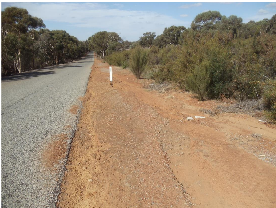
Poor drainage on southern side of road – note water damaging shoulder and lack of drain for water to flow down
