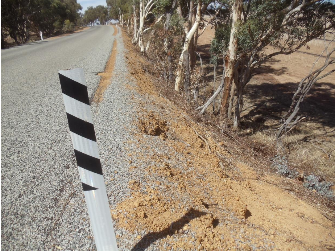
Looking east from southern side of the road - note narrow shoulder and steep batter. Note batter erosion
