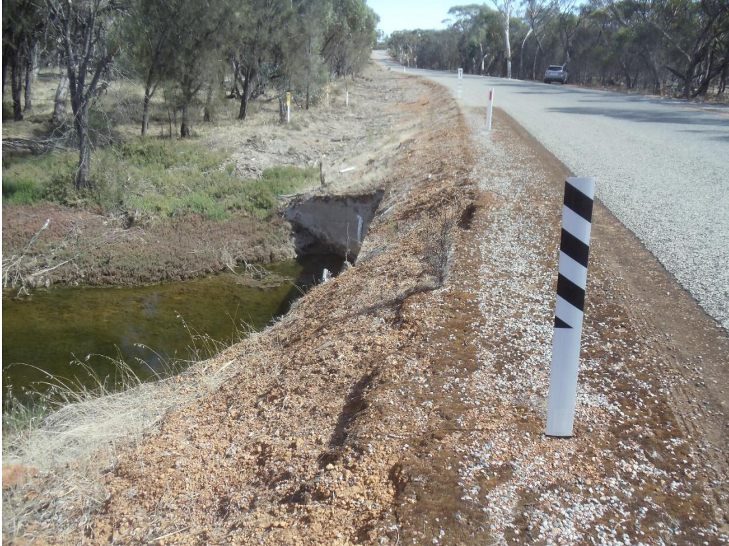
Shoulder on south side of road - narrow
