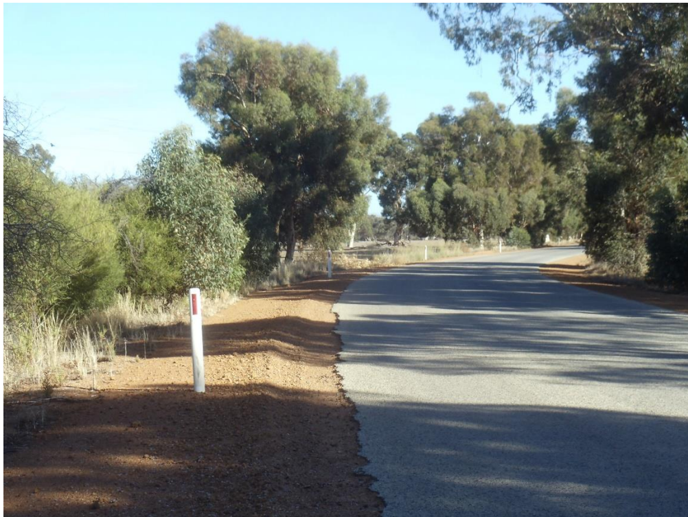
Note trucks running off road on outside of curve – narrow shoulder encroachment of vegetation. Note loss of seal edge. Vehicles can loose control on soft shoulders
