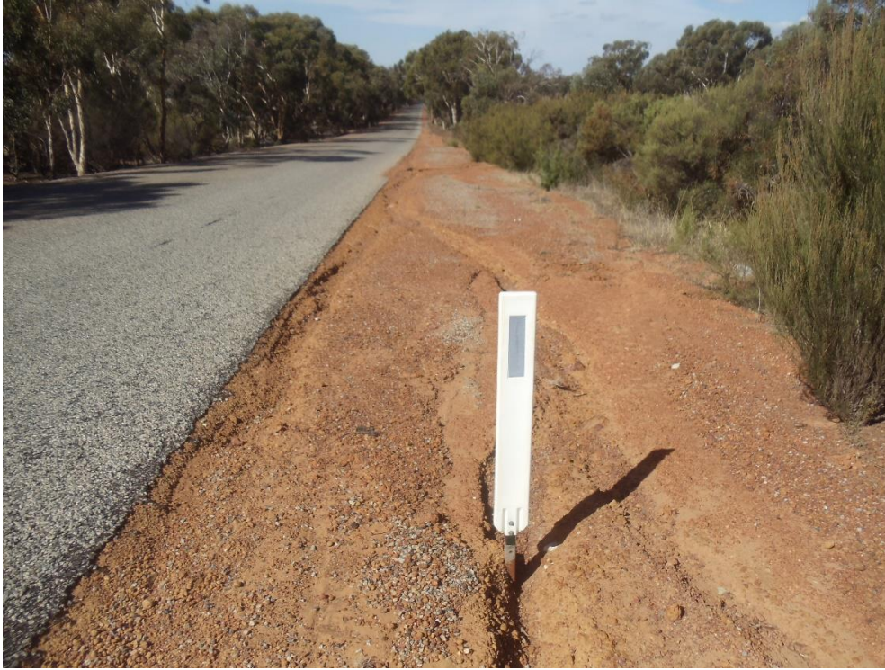
Poor drainage on southern side of road – note water damaging shoulder and lack of drain for water to flow down
