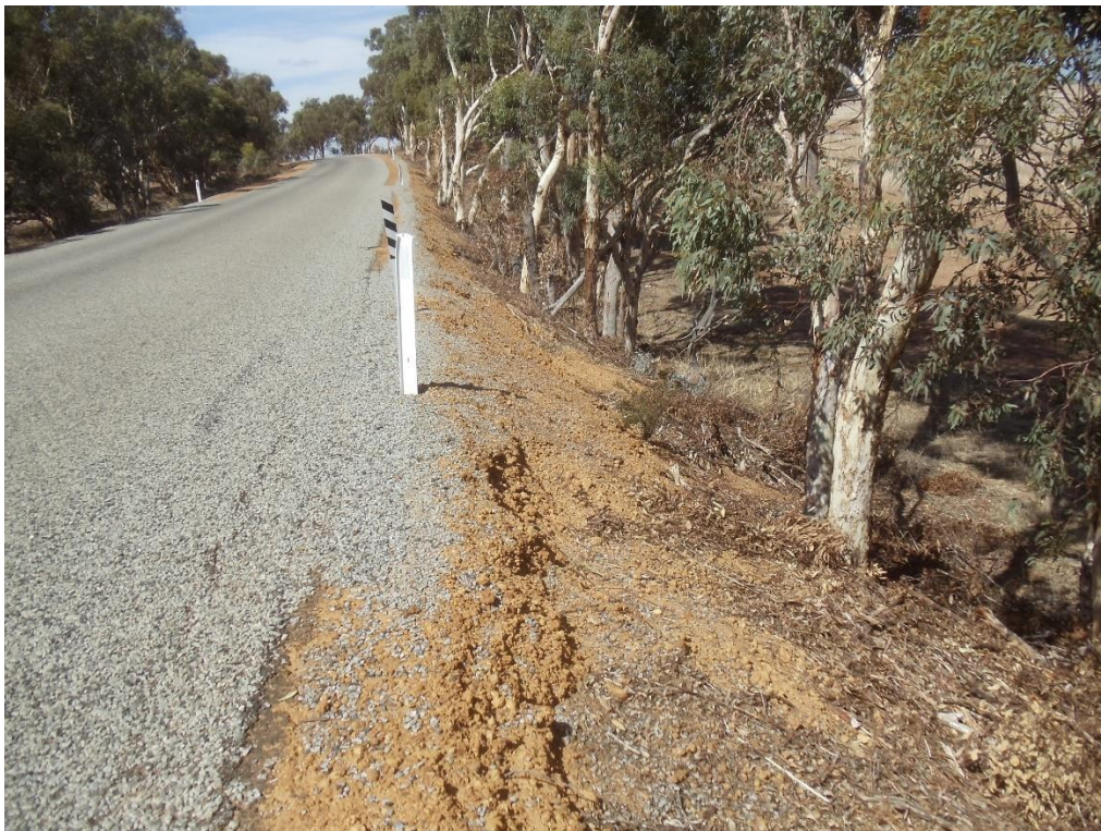
Looking east from southern side of the road - note narrow shoulder and steep batter. Note batter erosion
