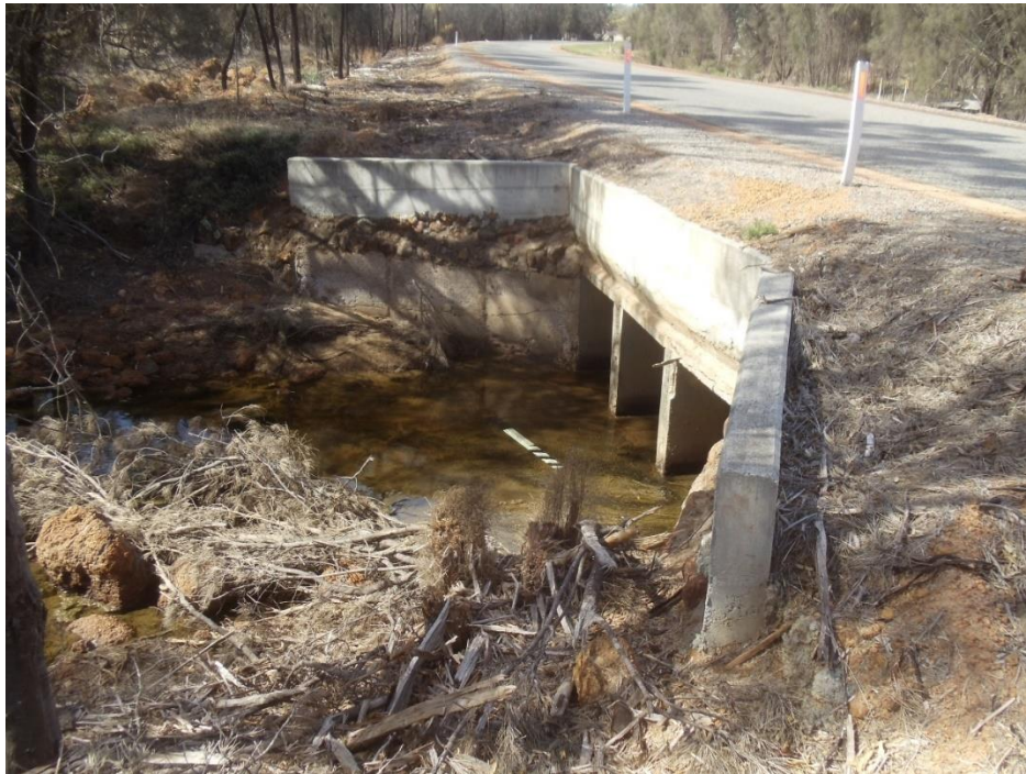
Culvert from north side of road – end of culvert too close to the road
