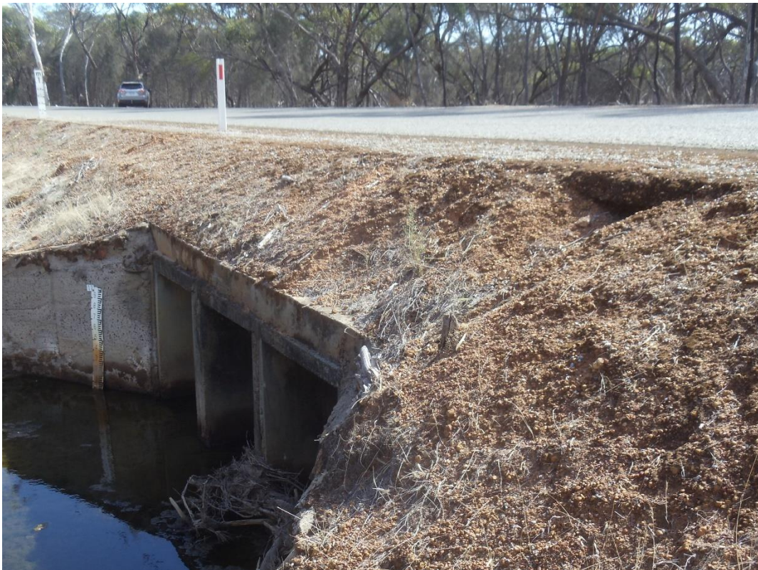
Culvert from south side of road – end of culvert too close to the road – sudden drop off
