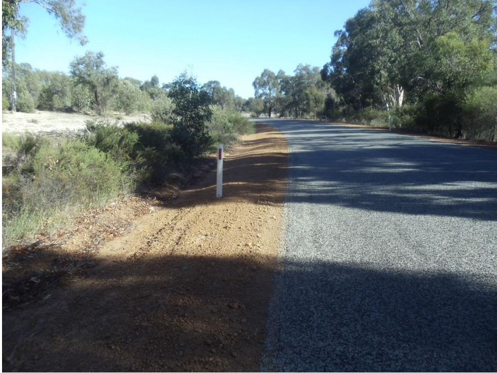
Note trucks running off road on inside of curve – narrow shoulder, encroachment of vegetation on right hand side
