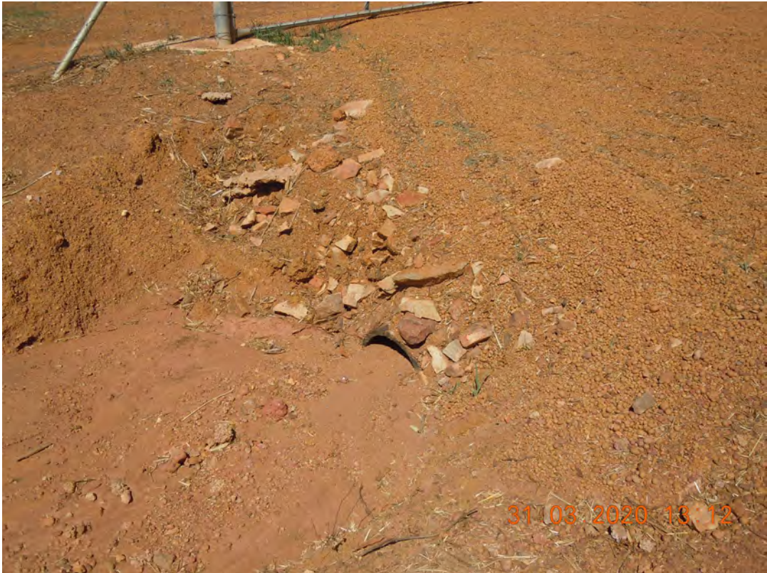
PHOTOGRAPH 5 - SLK 2.8 Cocking Road Downstream outlet of driveway culvert blocked
