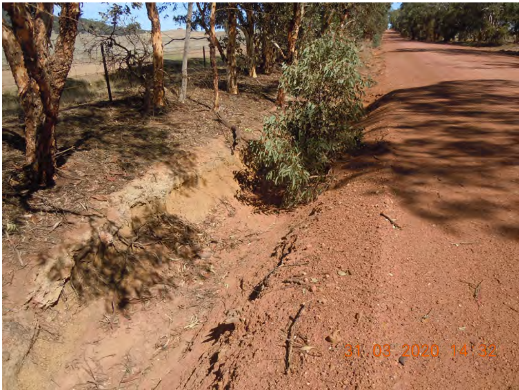
PHOTOGRAPH 24 - 0.29 SLK Cocking Road drain LHS
