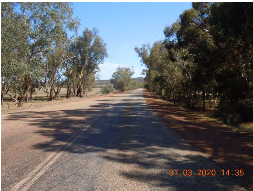
PHOTOGRAPH 4 - SLK 6.15 Mogumber Yarawindah Road looking west from Cocking Road Intersection- Typical View
