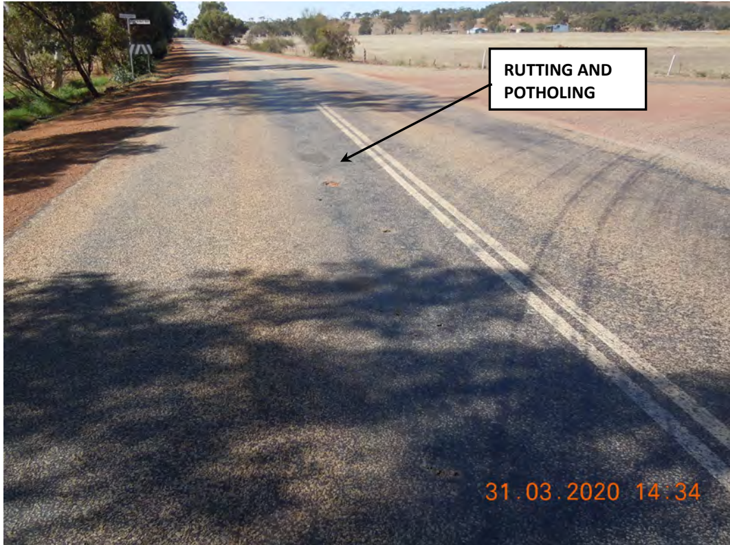
PHOTOGRAPH 26 - Mogumber Yarawindah and Cocking Road intersection Pavement Failure. Rutting and Potholing
