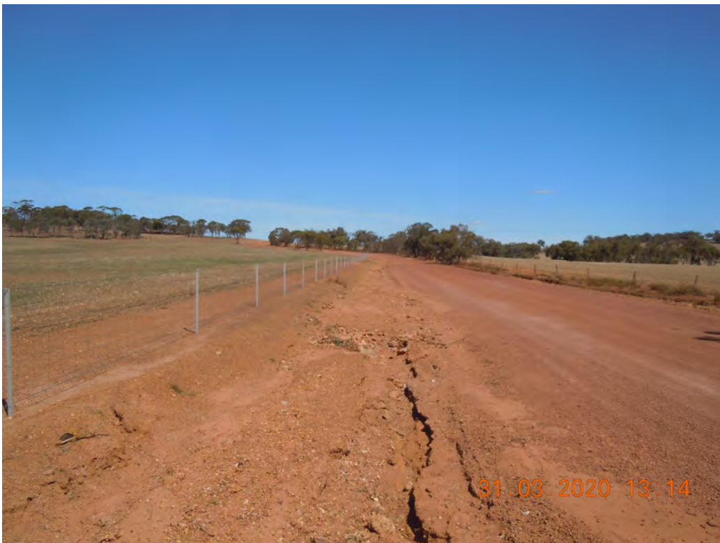
PHOTOGRAPH 6 SLK 2.8 Cocking Road Looking south scoured and debris filled drain
