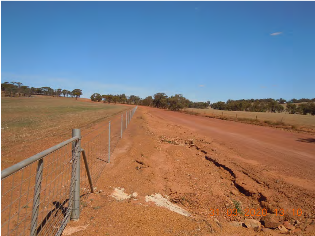
PHOTOGRAPH 3 - SLK 2.8 Cocking Road Looking south from proposed pit access road. Note scour and debris in drain
