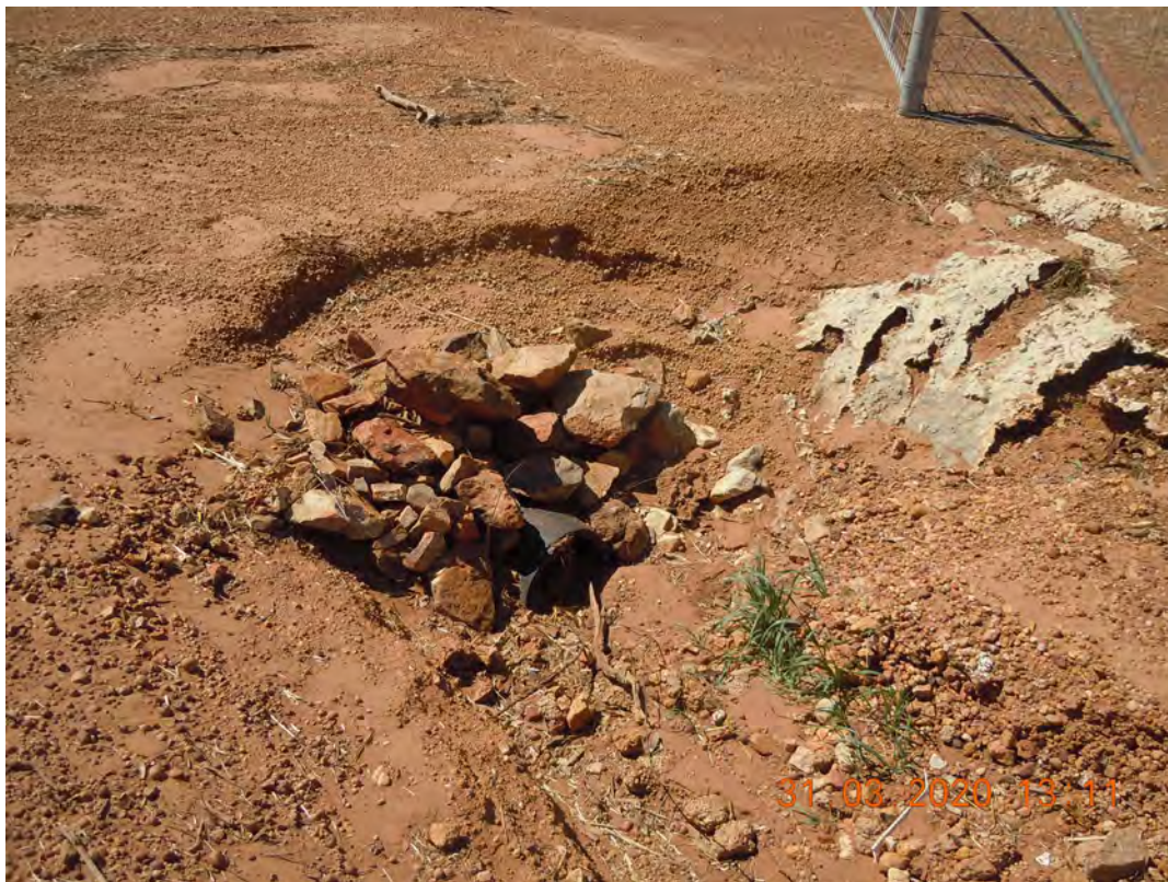
PHOTOGRAPH 4 - SLK 2.8 Cocking Road Upstream inlet of driveway culvert blocked
