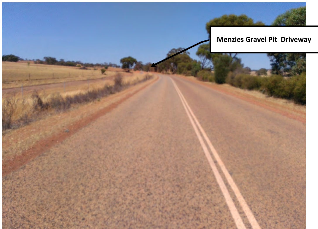
PHOTOGRAPH 4 8.19 SLK Looking West Can see driveway without looking over top of vegetation
