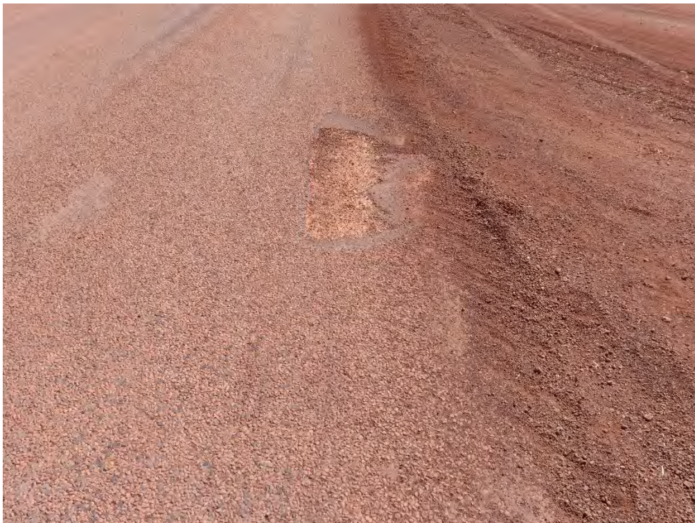
PHOTOGRAPH 6 7.95 SLK Seal damage at Menzies Pit Driveway on Mogumber Yarawindah Road
